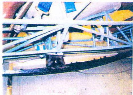
Top: the nosewheel, a modification signed off in June 1985, will absorb impact energy but also cause rebound. Bottom, the skid's rubber mounting block, directly under the front seatpan, will transmit impact loads up the spine.
